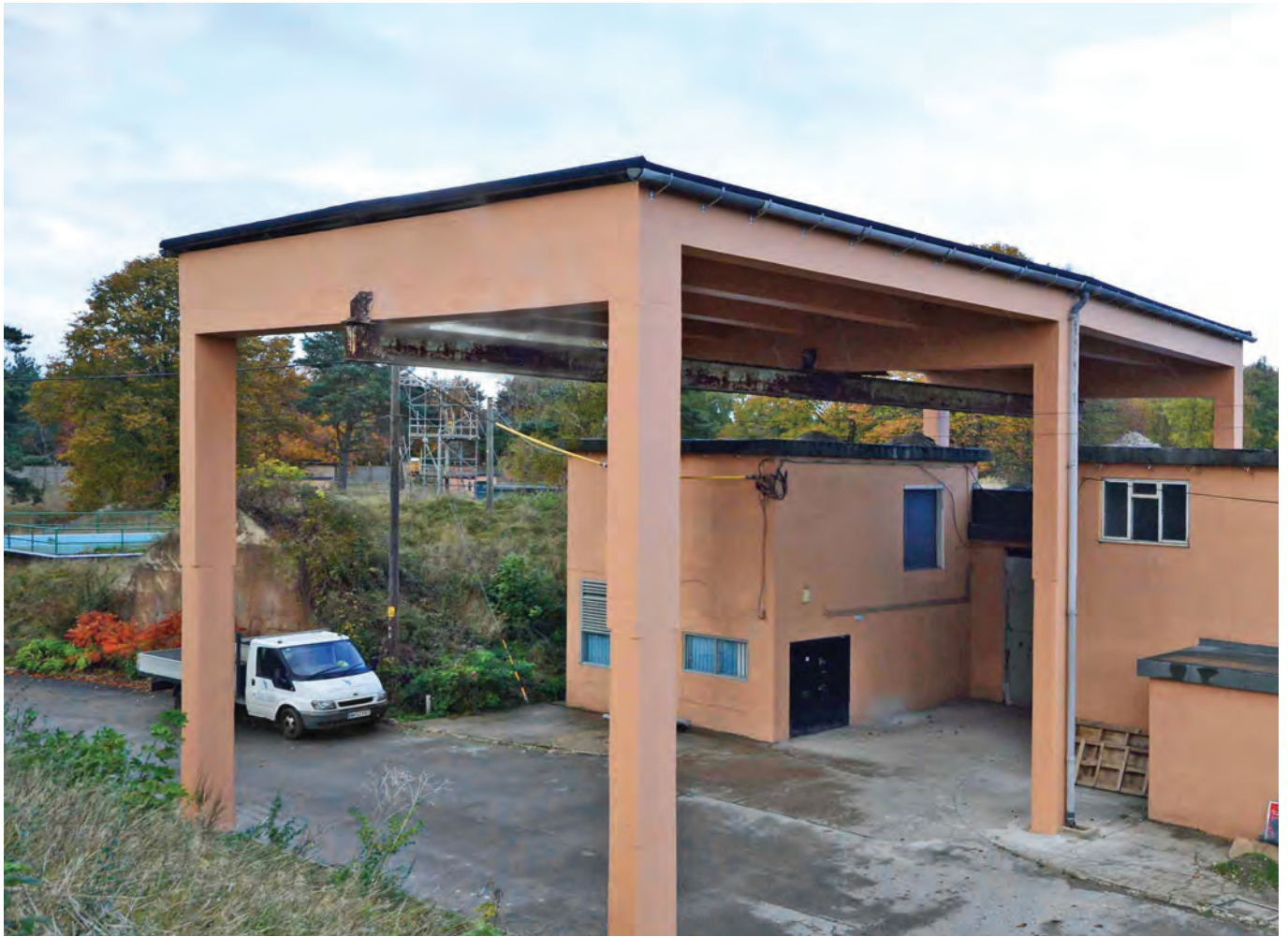
Non-nuclear Component Building 60 and its refurbished gantry seen from the opposite berm. The steel joist runway beam for the hoist can be seen
